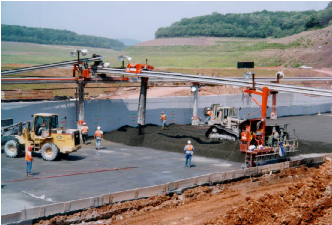
Figure 6-2. Conveyor system with mobile side discharge belt
